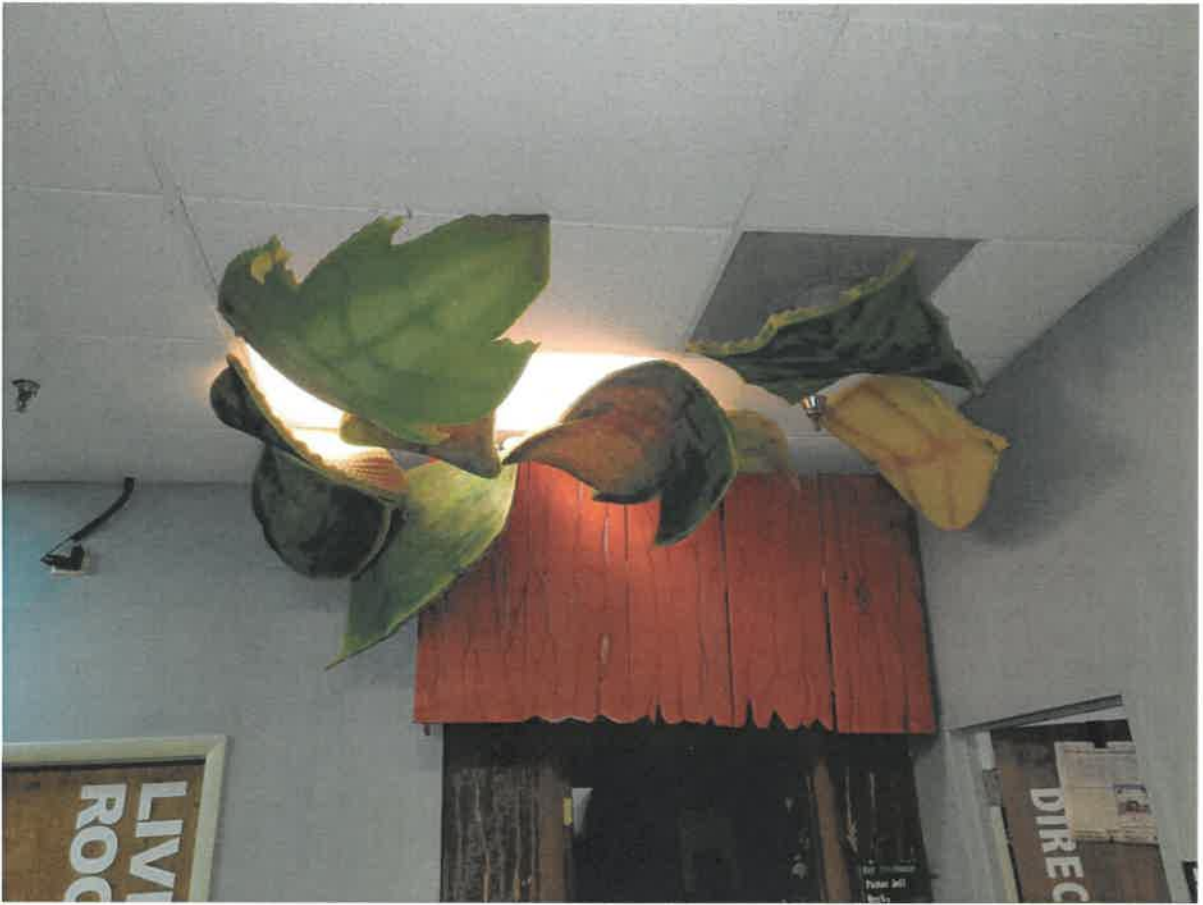
FOAM LEAVES ON CEILING NEAR SPRINKLER HEAD SUITE 103 – PHOTO TAKEN 3-14-23
