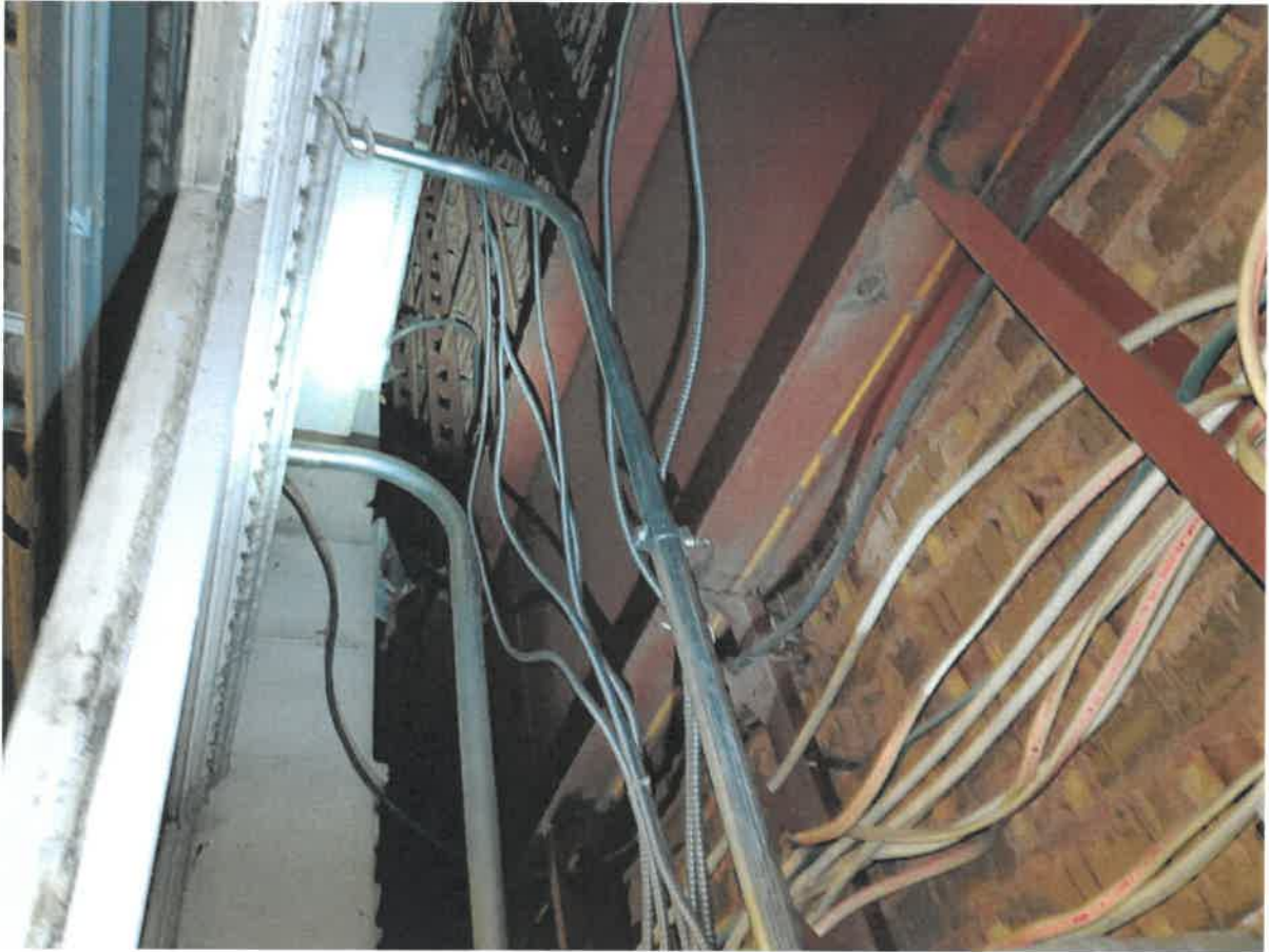
ELECTRIC PANELS INSTALLED ON THE BRICK FAÇADE – M&T SIDE – PHOTO TAKEN 3-14-23
