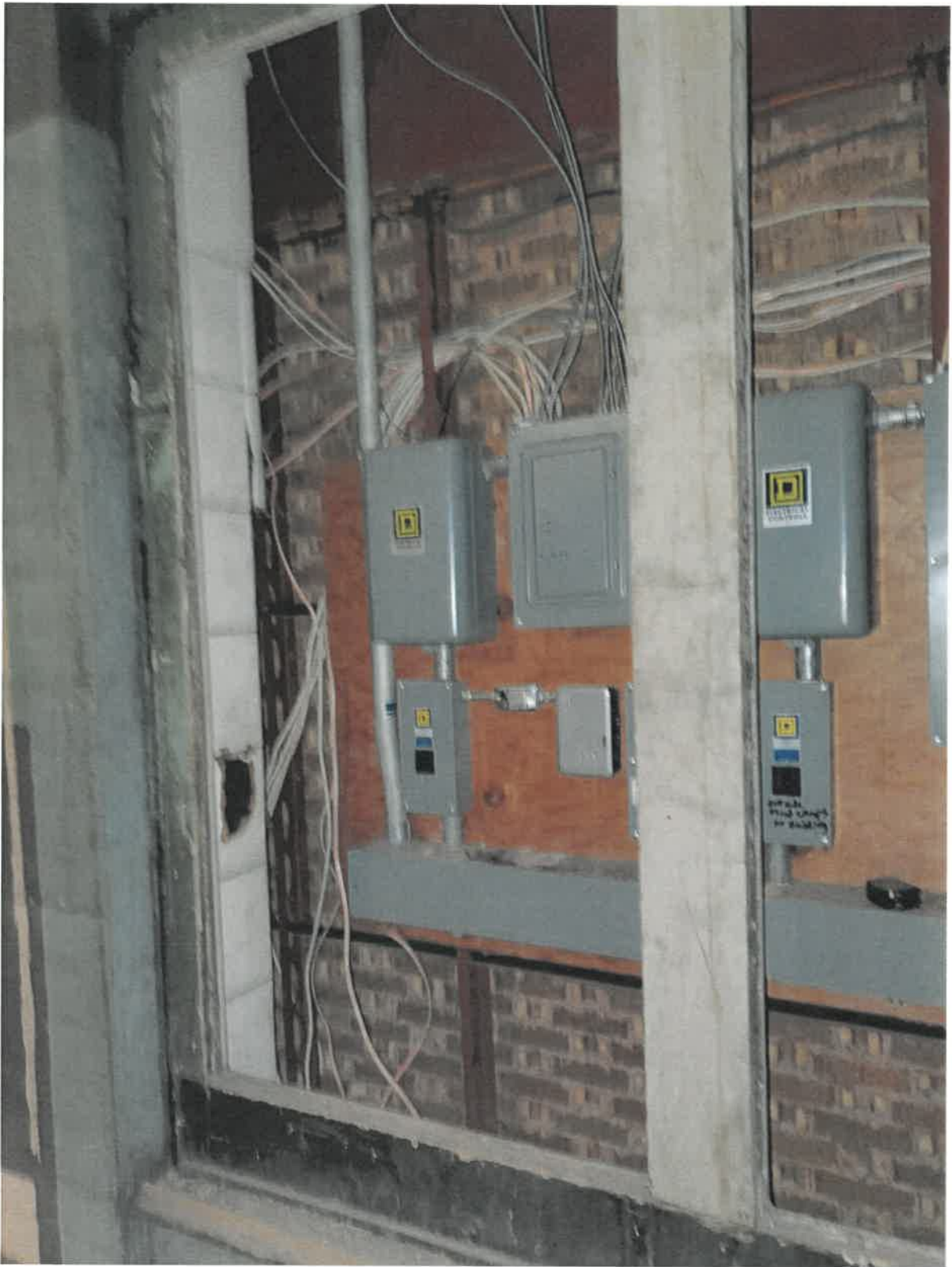
ELECTRIC PANELS INSTALLED ON THE BRICK FAÇADE – M&T SIDE – PHOTO TAKEN 3-14-23
