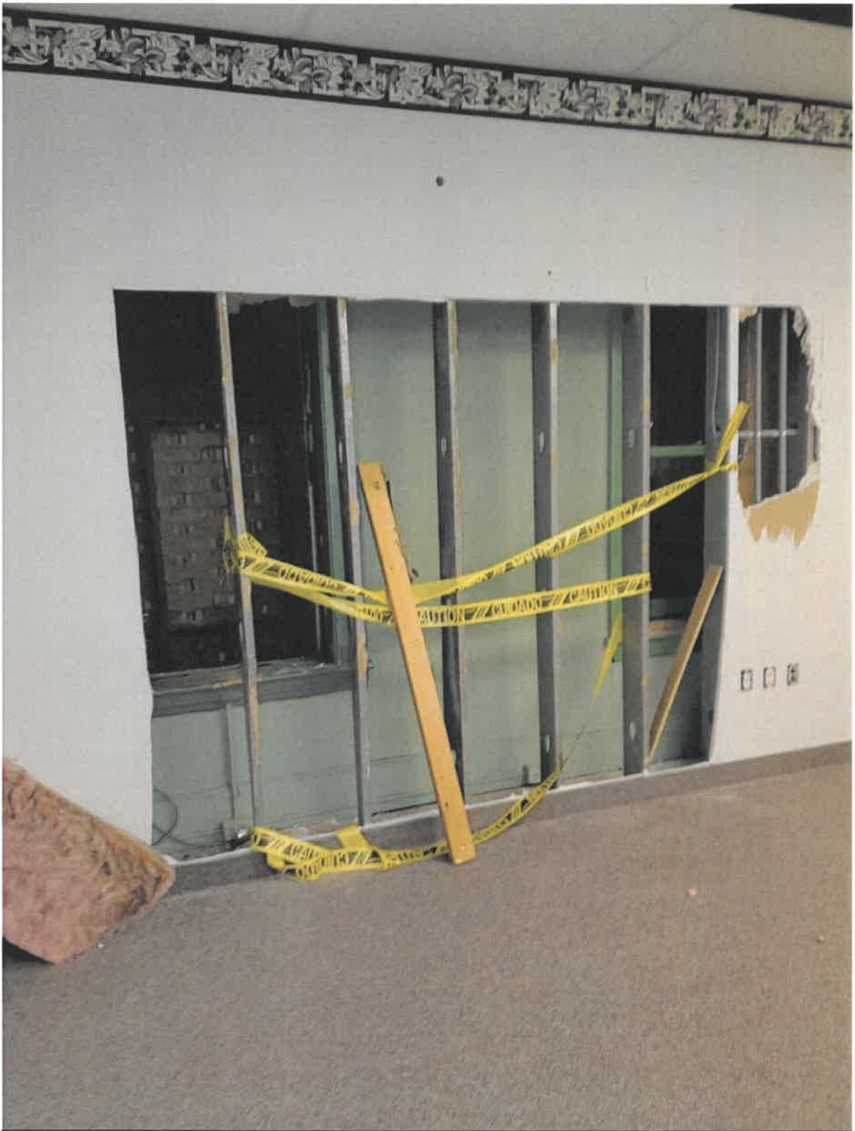
M&T BANK WALL OPENING – PHOTO TAKEN 3-14-23
