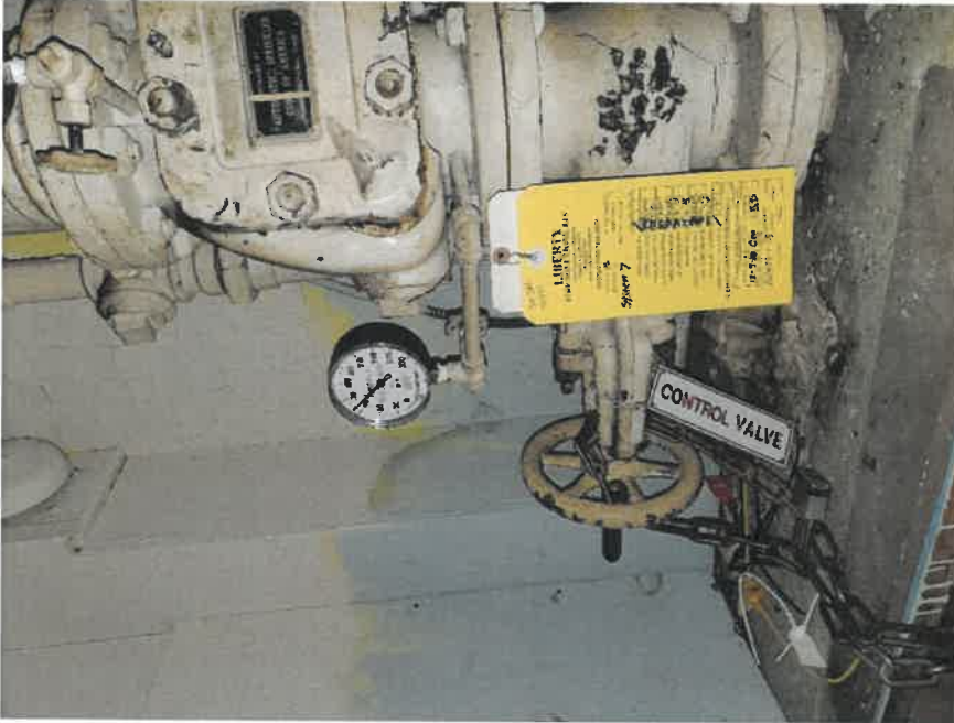
GAUGE AND STEM AND YOLK VALVE LOCKED IN THE OPEN POSITION
