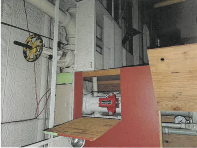
RISER #2 - PRESSURE SWITCH
