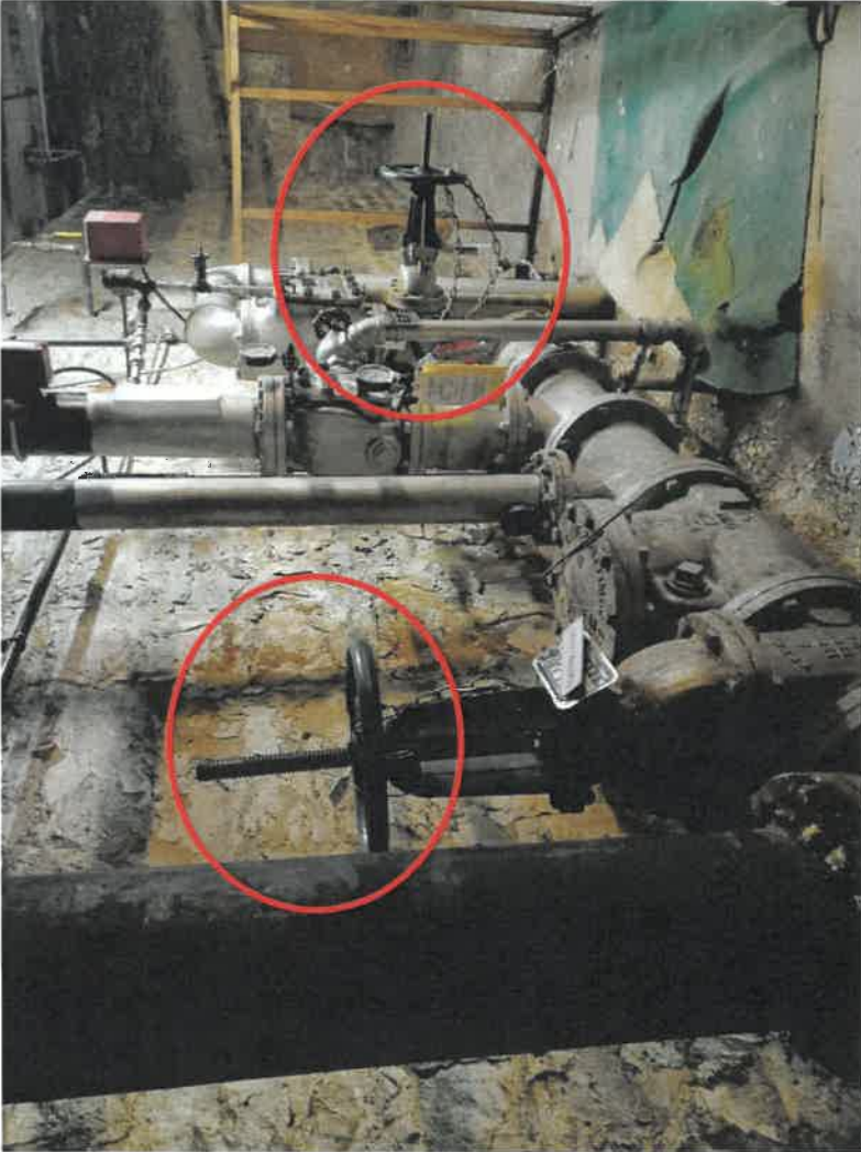
RISER #5 - BASEMENT GAME ROOM - STEM AND YOLK VALVE OPEN
