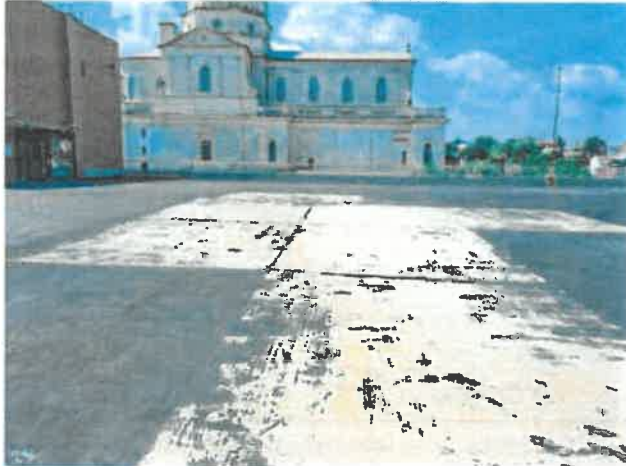
Photo 13 – Top Level failed traffic topping
