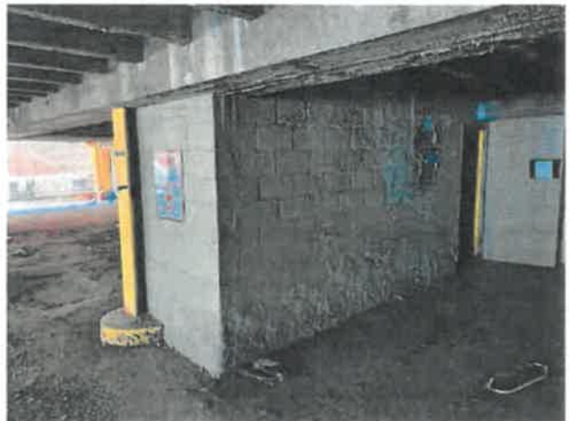
Photo 24 – Failed stair and tower
