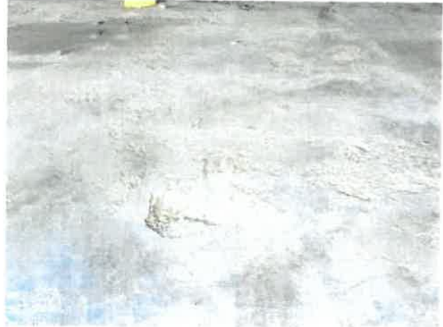
Photo 28 – Typical spalled floor slab
