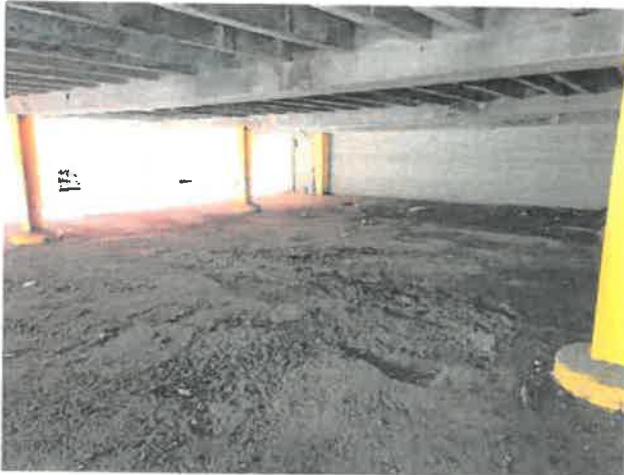
Photo 27 – Typical spalled floor slab
