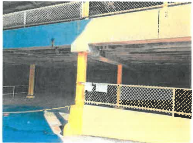
Photo 30 – Perimeter restraint require vehicle upgrade
