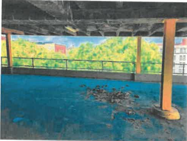
Photo 19 – Loose Failing Concrete
