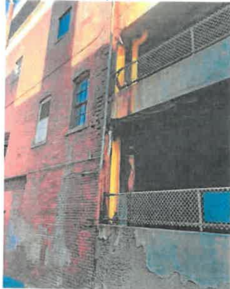
Photo 4 – Typical façade Deterioration
